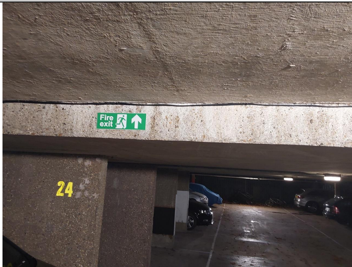
Fire exit signs in garage
