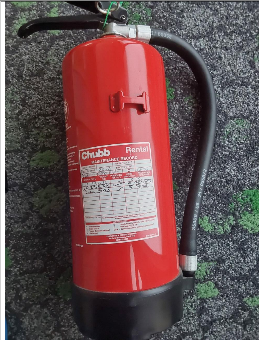
Remaining extinguishers tested 9/24
